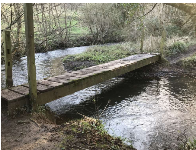
Figure 25 – Footbridge at entrance G. Note steps at ends and lack of handrail
