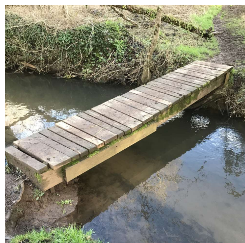
Figure 26 – Footbridge at entrance F. Note repair to beam, lack of handrails, bank erosion and steps at each end
