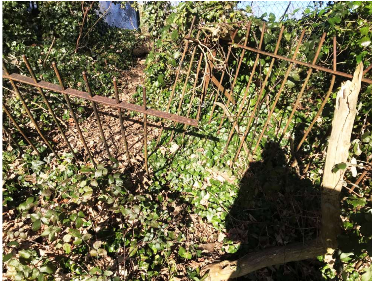
Figure 30 – damaged railings to college site by the central pill box
